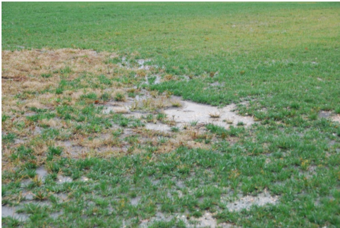
Surface ponding due to compacted soil.
